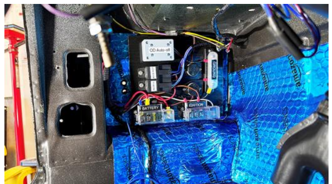
Aux Electrics Panel
